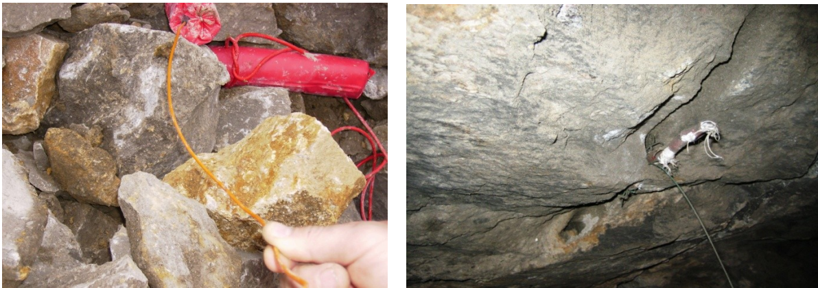
Figure 2: Rest of explosives in muck pile, surface (left) and in trim-holes, underground (right)
